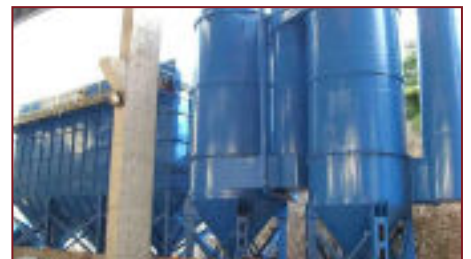
Mechanical vibration dust collector
