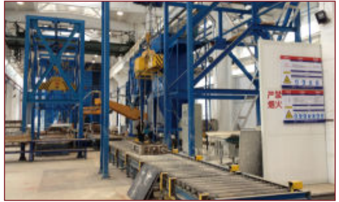
Resin Sand Reclamation Production Line
